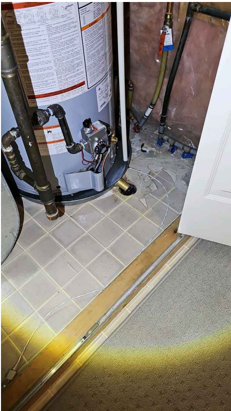
Floor drain: Location Near water heater
