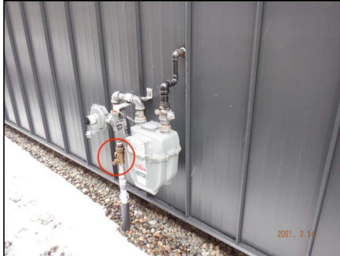
25. Main Fuel (GAS) shutoff
