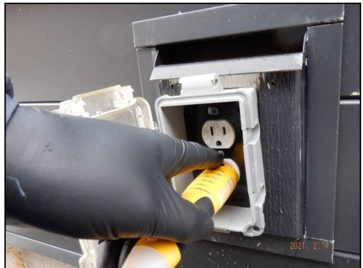
24. GFCI/GFI needed (Ground Fault Circuit...
